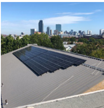
Tobin Community Center solar installation.
