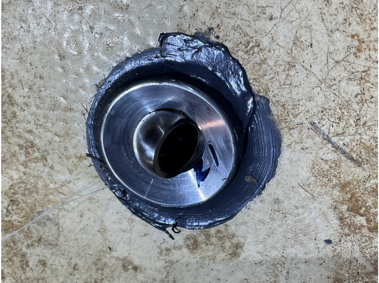
Close-up photo of a newly installed transducer used to determine the flow rate
