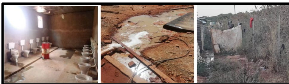
The images above show the workers’ bathroom, open sewage, and a worker bathing in a makeshift facility at Arcadia Mine (Mary Taruvinga/NewZimbabwe). 230
