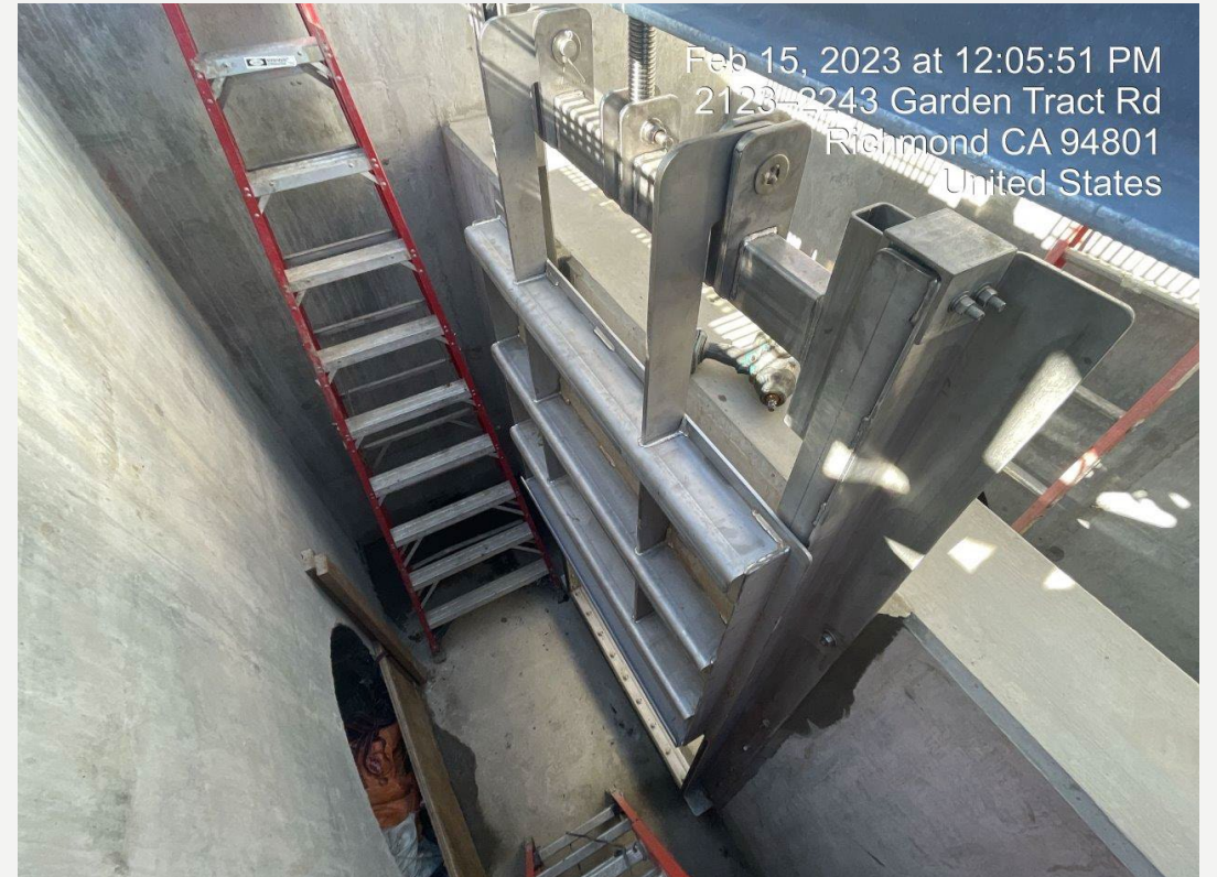
Sluice gate between existing EQ Basin I and new EQ Basin 4
