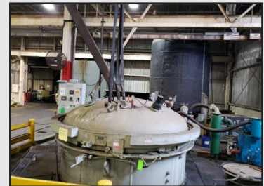
HEATTEK VPI SYSTEM
