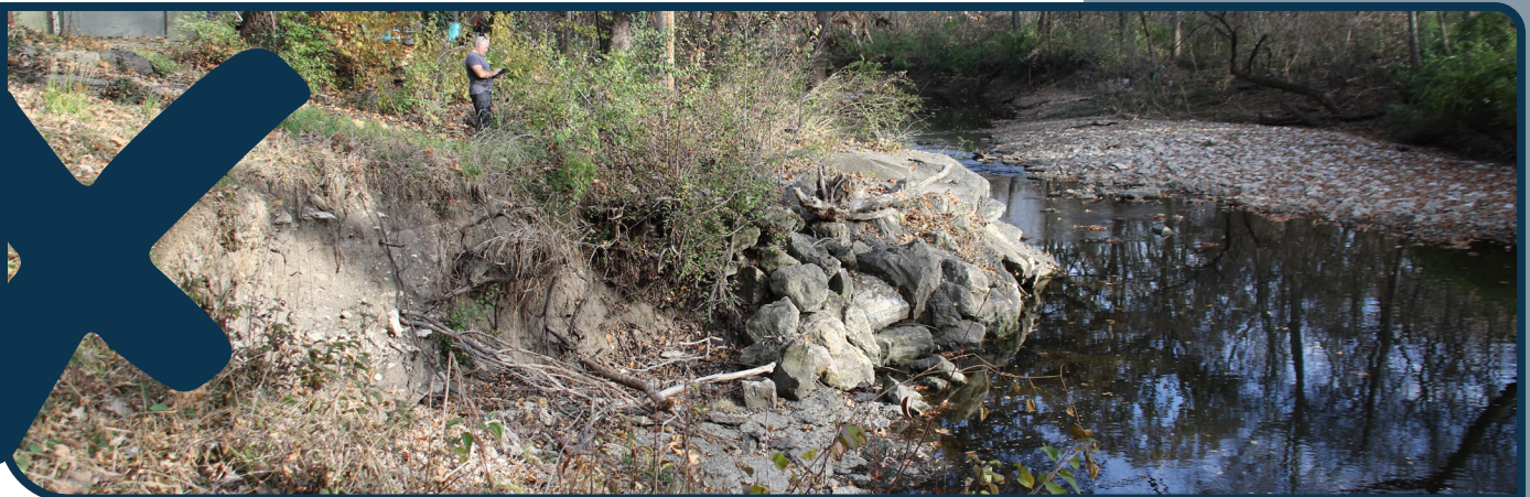
Severe streambank erosion
