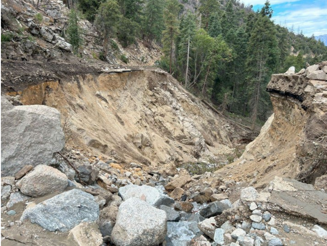
Postmile 23.90 embankment/roadway washout
