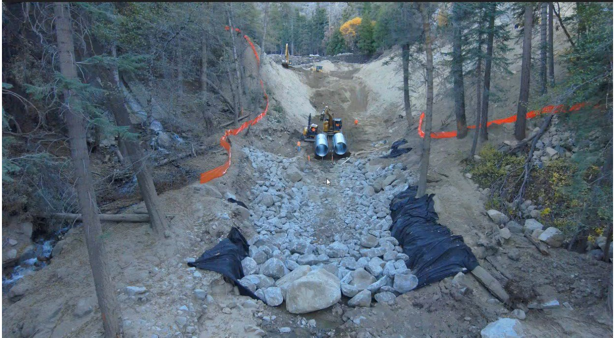
Postmile 23.90 embankment/roadway washout
