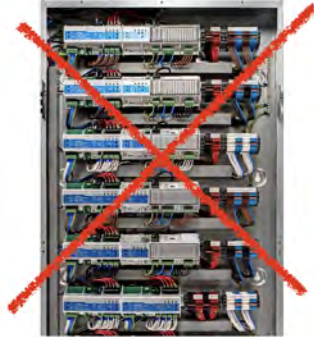
No Control Cabinets
