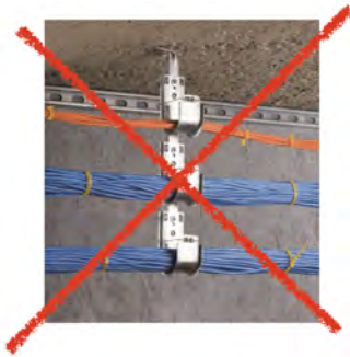
No Control Wires
