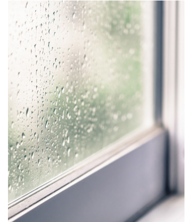
When humidity is not controlled, condensation can form on windows.
