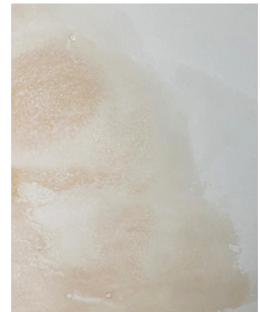
Ceiling stains can be a sign of uncontrolled humidity.
