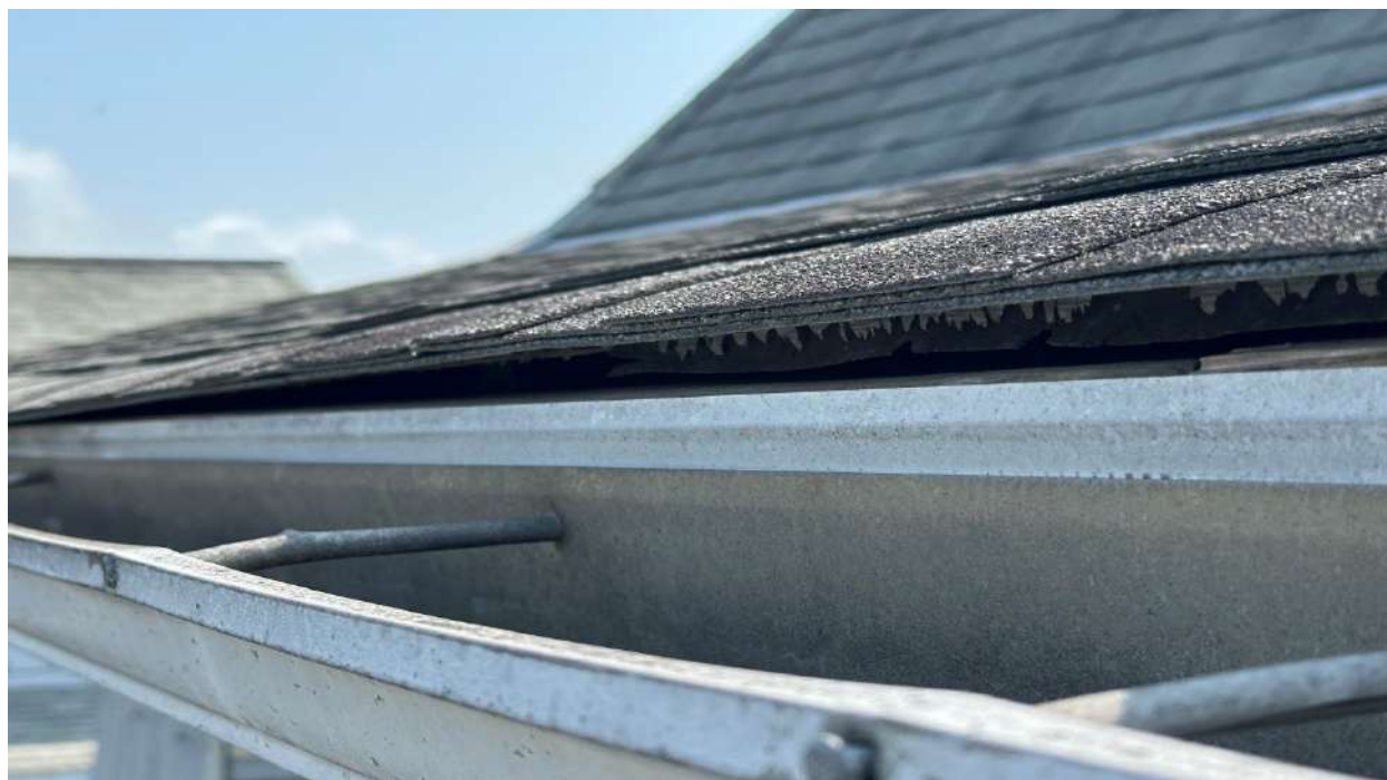
P-52 Gap at Shingle at Gutter exposing Sheathing
