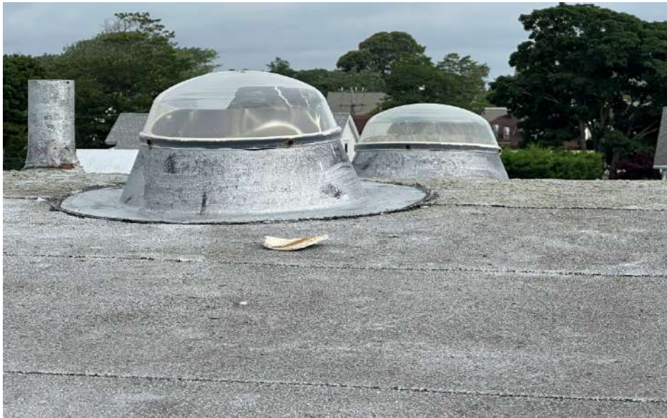
P-6 Solar Tube Skylight
