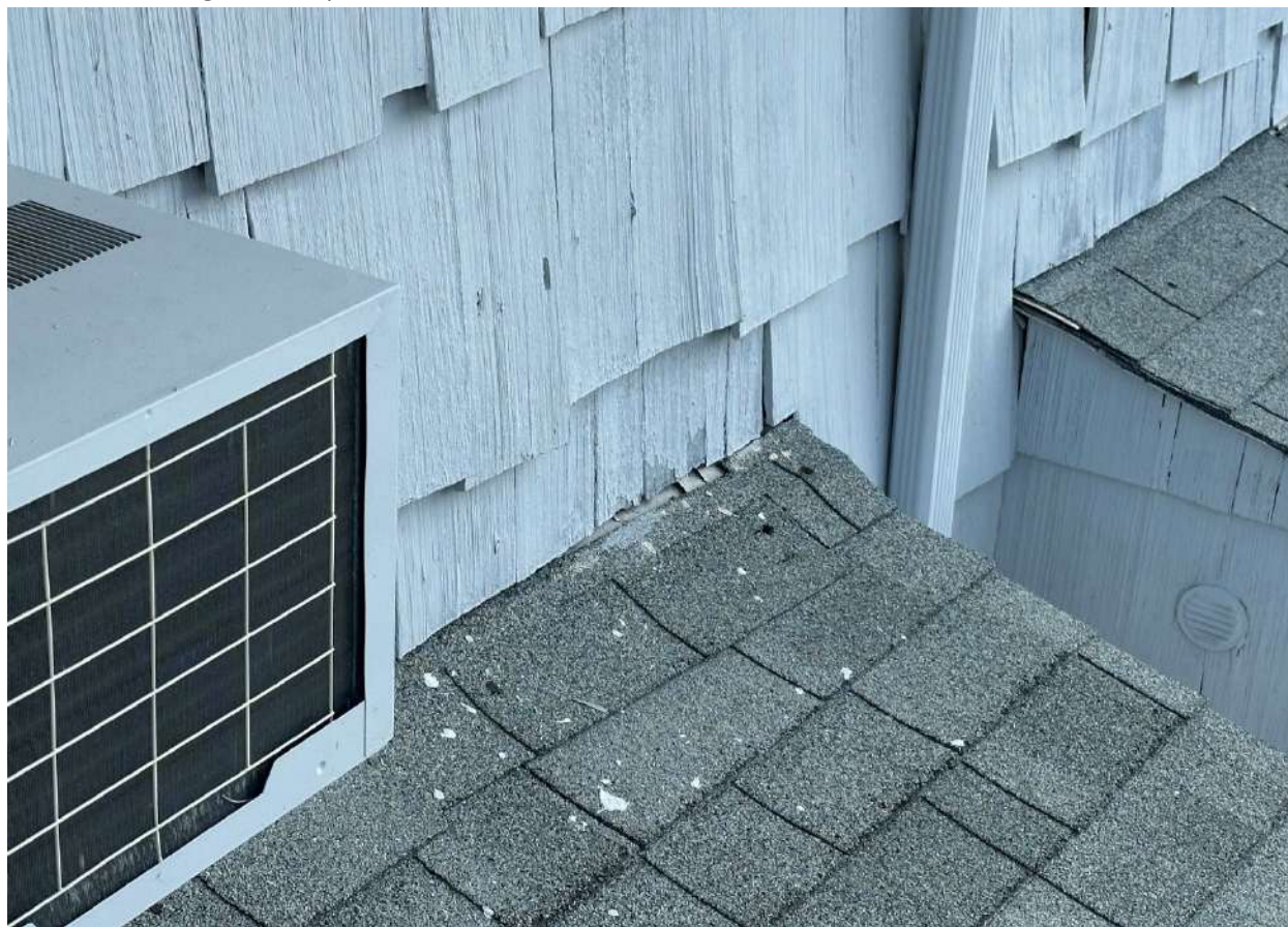
P-51 Loose Shingle and Exposed Fasteners
