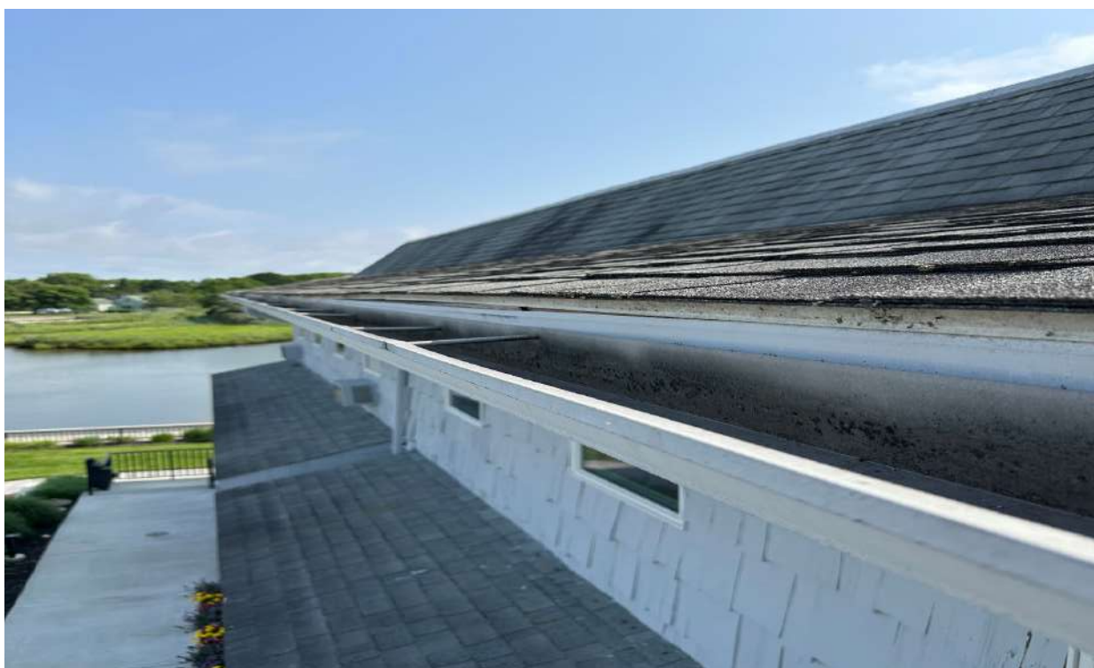
P-64 Gap At Shingle At Gutter Exposing Sheathing
