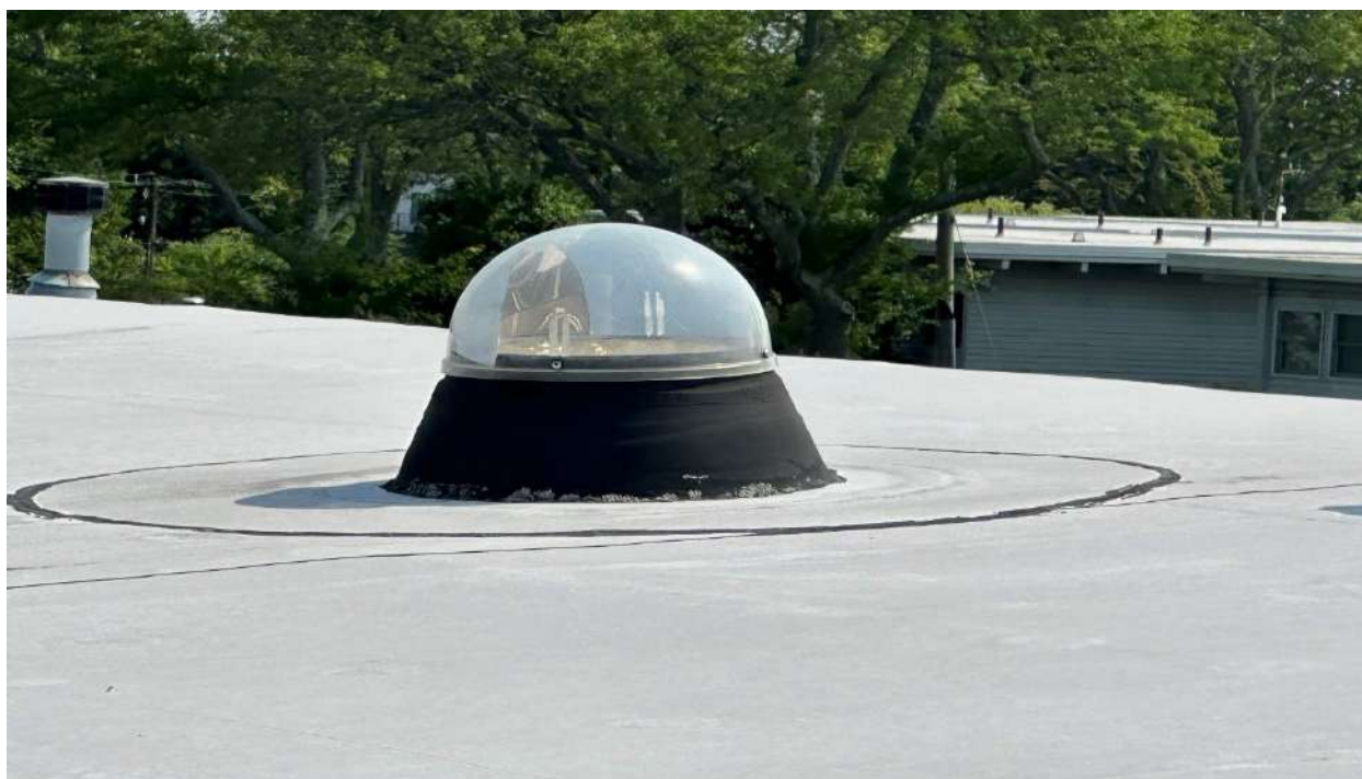
P-56 Solar Tube Skylight With TPO Flashing
