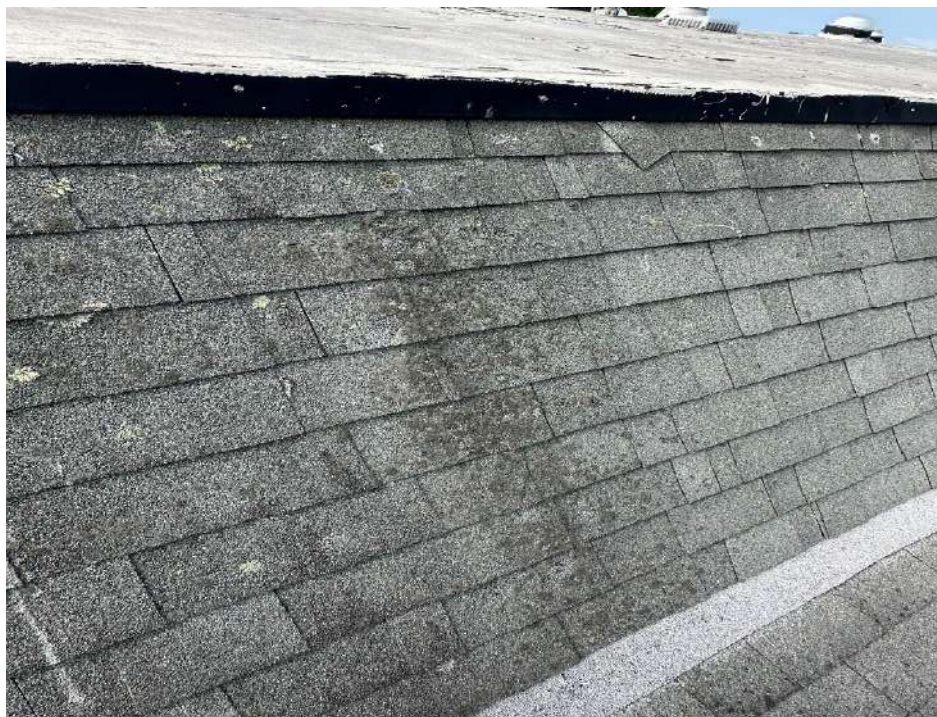
P-44 Delaminating Shingle
