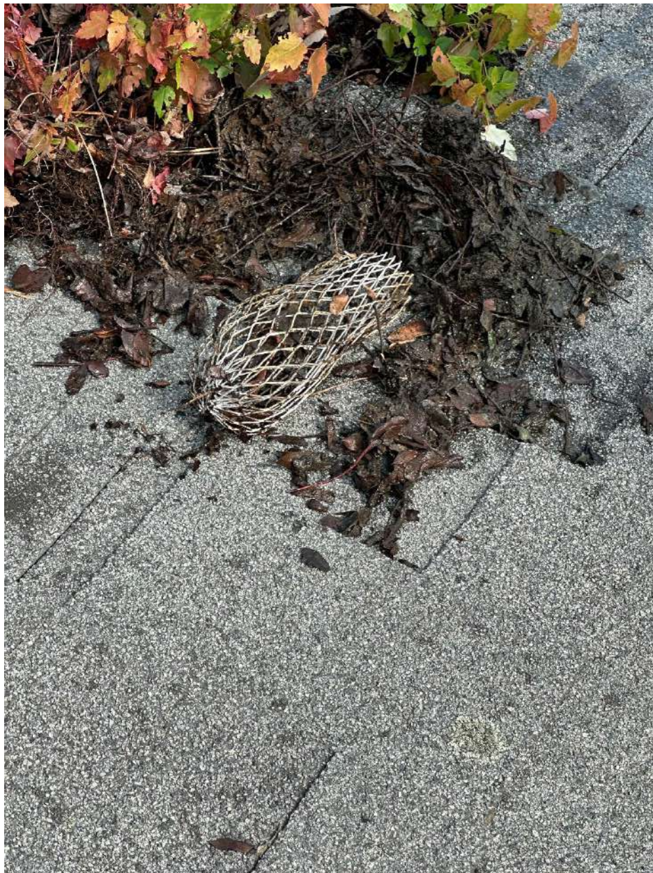
P-48 Strainer in Gutter at Leader Opening
