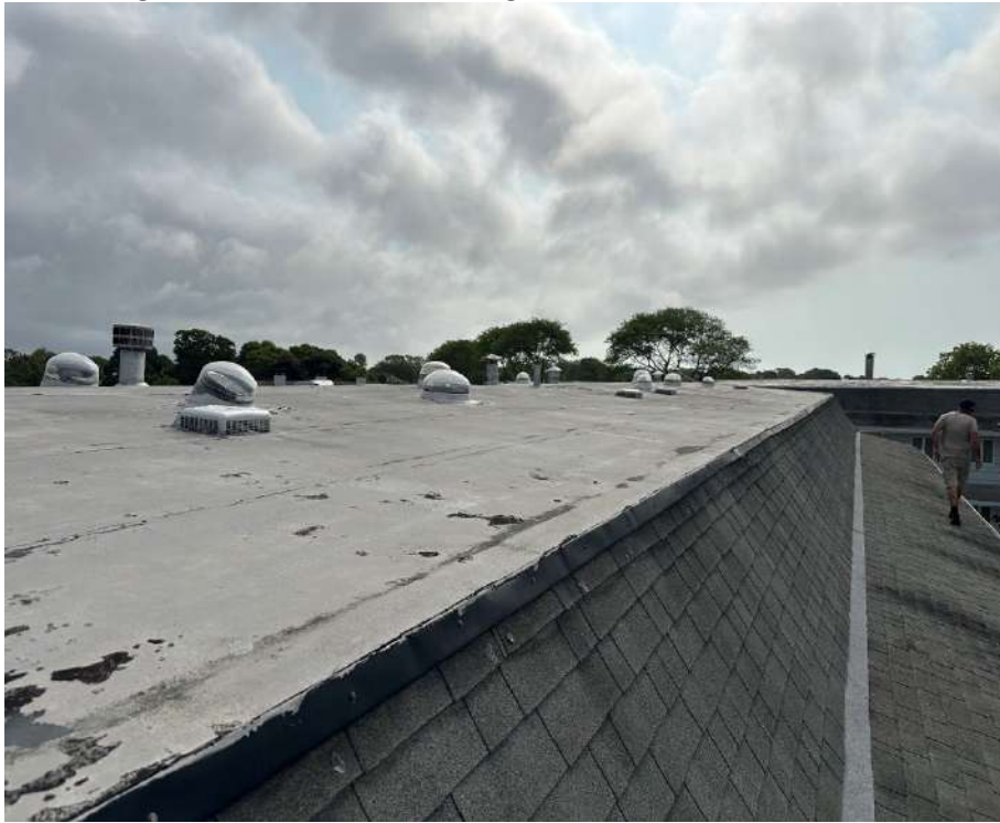
P-8 Peeling Fibrated Aluminum Coating
