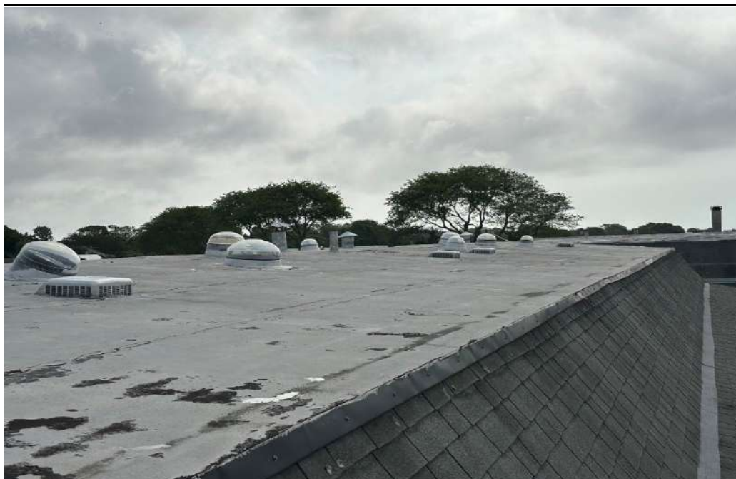
P-17 Gap at Fascia Exposing Sheathing
