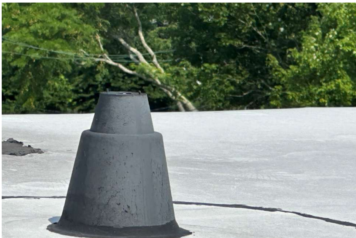
P-60 Relief Vent Cap Missing
