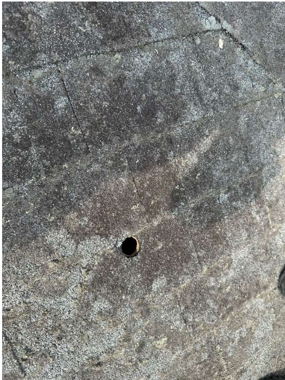
P-33 Hole Drilled Through Roof
