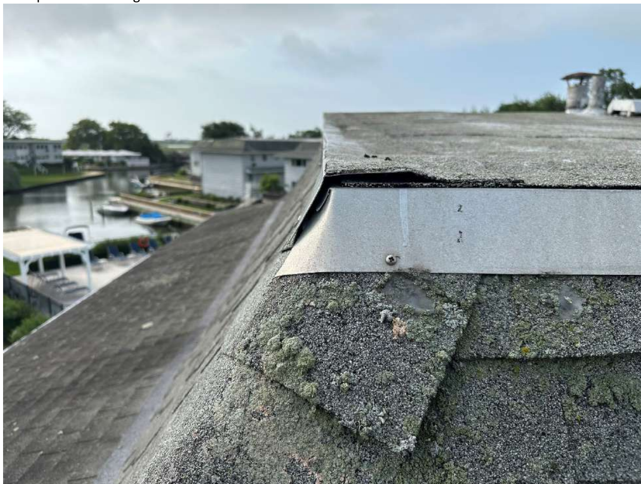
P-5 Open Seam At Edge Metal
