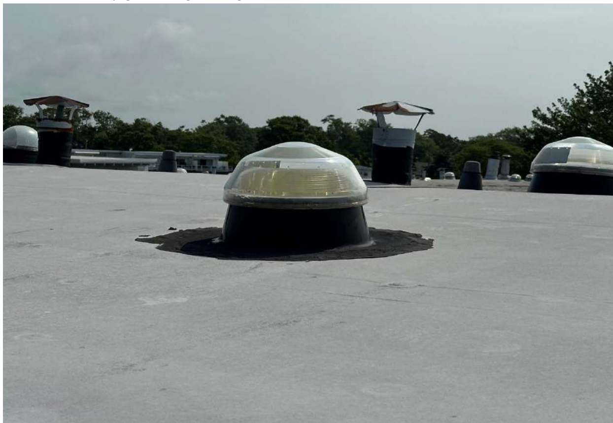
P-55 Solar Tube Skylight Missing Flashing With Tar
