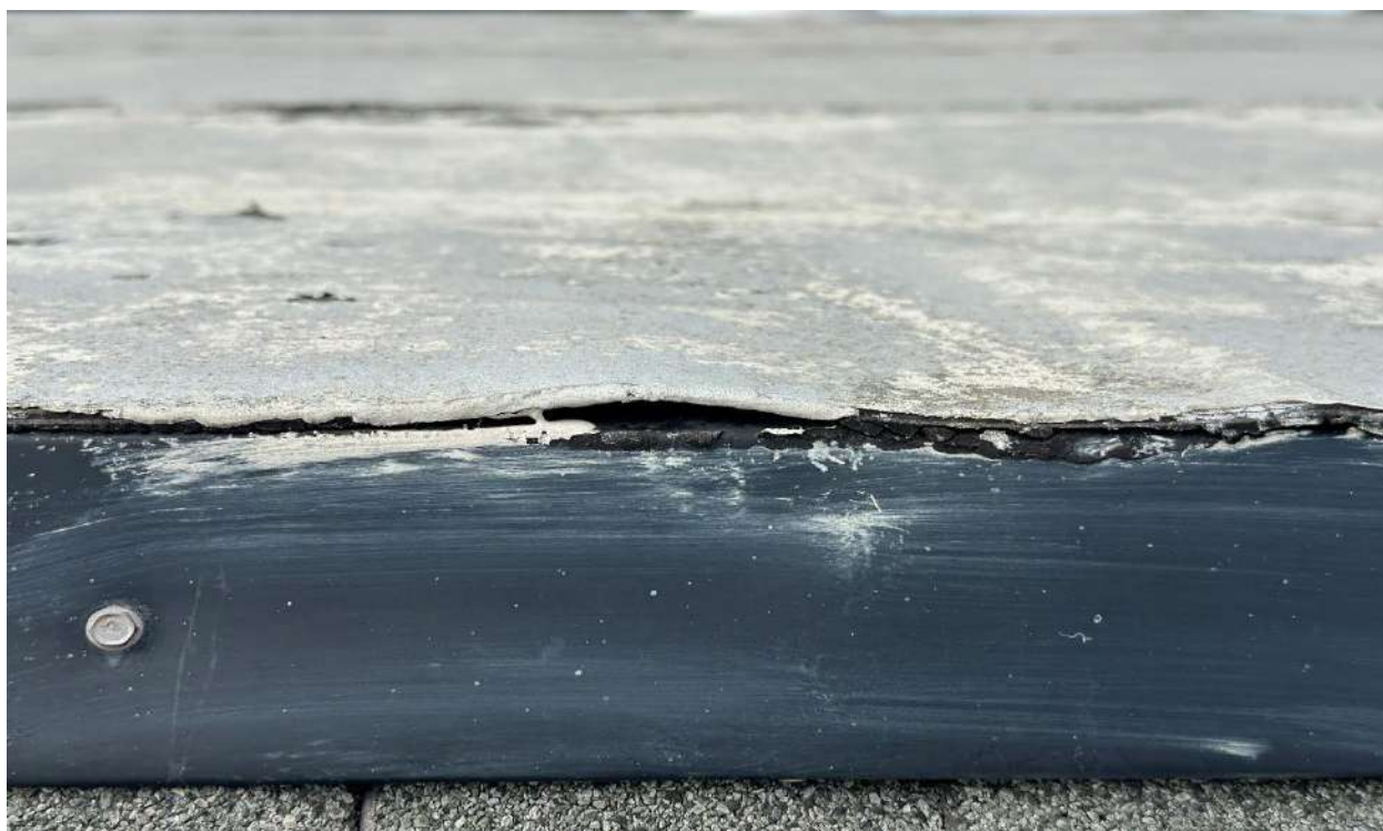
P-16 Peeling Fibrated Aluminum Coating
