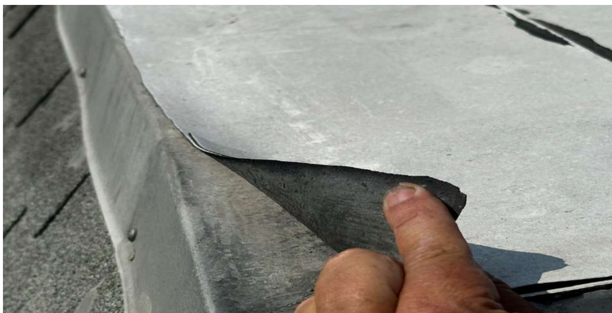
P-62 TPO Delaminating From Edge Metal
