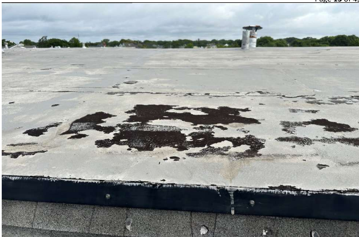
P-15 Opening in Membrane at Edge Metal
