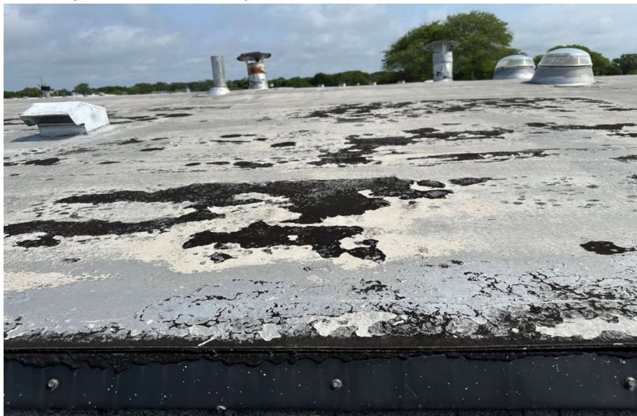
P-79 Peeling Fibrated Aluminum Coating
