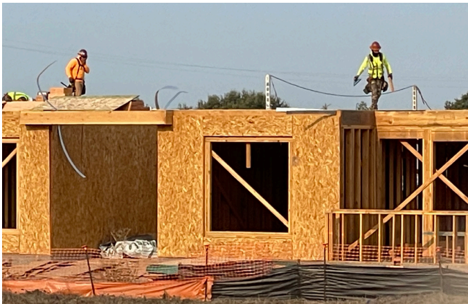
A residential construction project along Franz Kafka Ave. in Santa Rosa. Members of the industry say they are in a Kafkaesque situation with a Fed-OSHA demand that they adhere to a six-foot fall-protection trigger.
