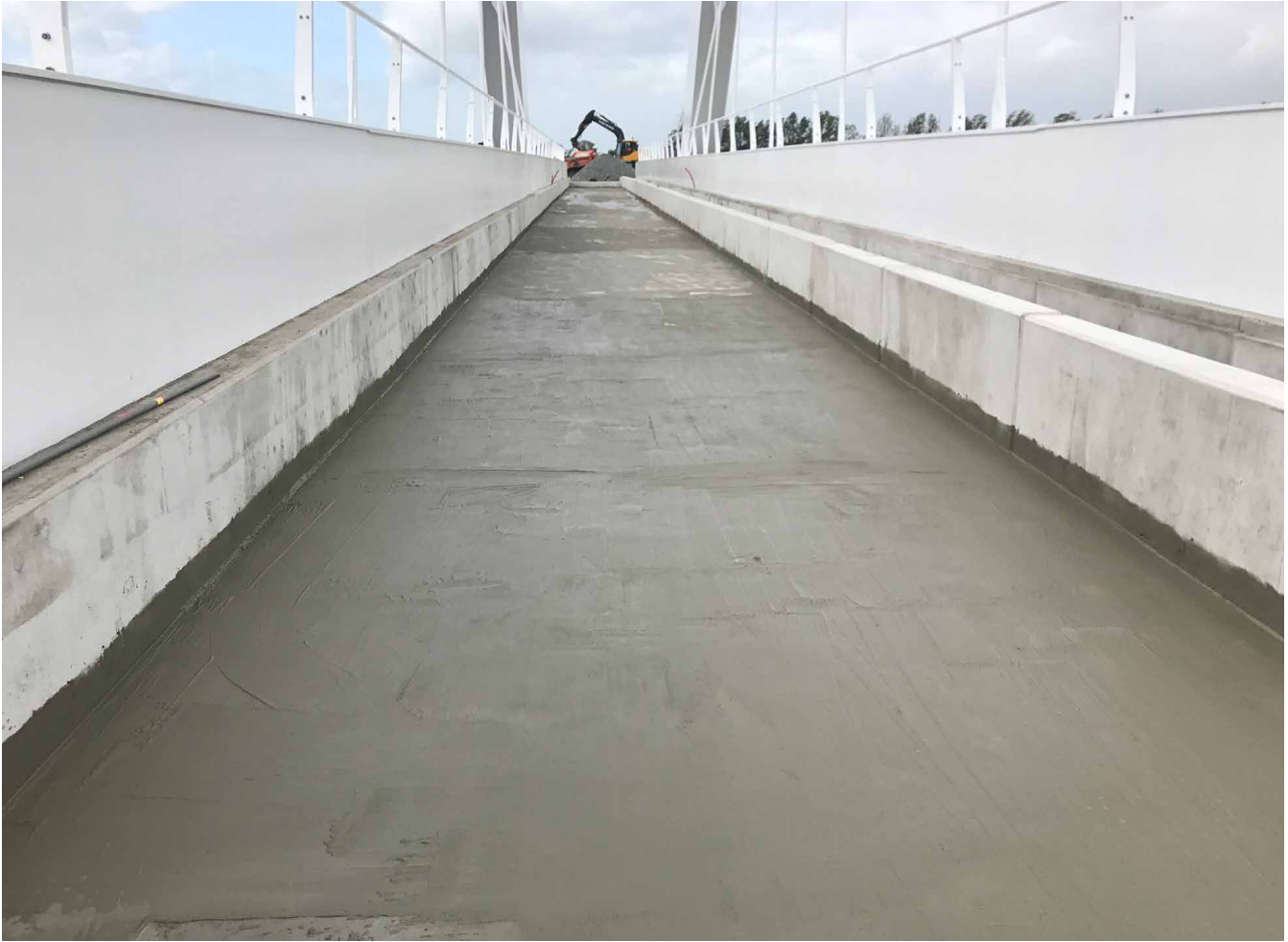
Fig 7 -- Xypex Conenstrate has been applied to the concrete deck of the new Zuidhorn railway bridge, creating a integral bond and protect the concrete from moisture and harsh chemicals.
