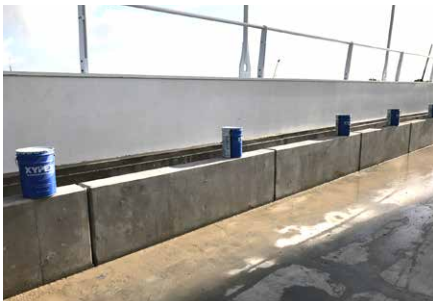
Fig 4 -- Buckets of Xypex Concentrate are pre-positioned along the concrete rail bed that lines the new Bert Swart Bridge in Zuidhorn, Netherlands.
