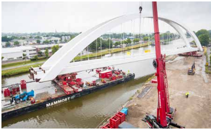
Fig 2 -- As assortment of heavy lift technology is employed by the Mammoet company in order to move one end of the 1,700-ton steel bridge across the canal and into its final position.
