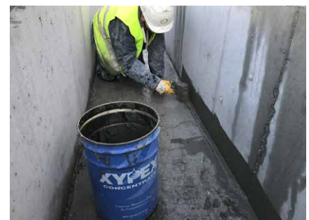
Fig 6 -- A Totech technician applies Xypex Concentrate with a stiff bristle brush along a walkway incorporated into the new Zuidhorn railway bridge.
