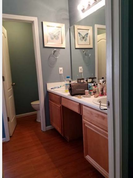
Outdated cabinets with inconvenient storage space
