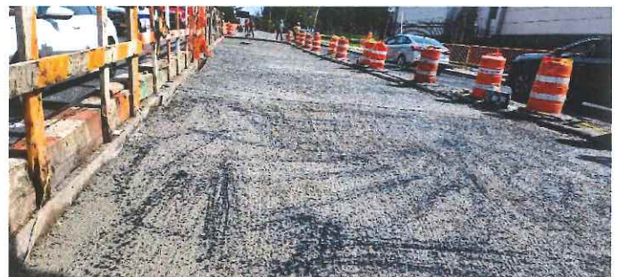
Roadway Base Concrete at East of Intersection of Jerome Ave. & E. 233 rd . Street
