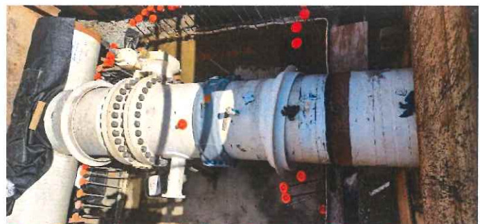
36-inch Trunk Water Main Butterfly Valve at Phelan Place
