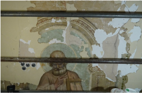
Saint Thomas—Restoration of S. Thomas' original halo. Note the loss of plaster, and consequently parts of Leduc's original mural, around him.
