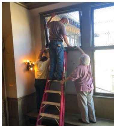
WSU carpenters and Freer House board member, Doug Peters, install a restored leaded glass window
