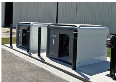
Electric aircraft charging infrastructure installed at Kissimmee Gateway Airport.
