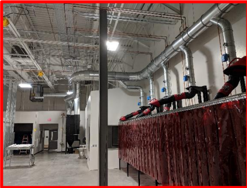
Picture 1: Duct Work and New Curtains in the Welding Lab
