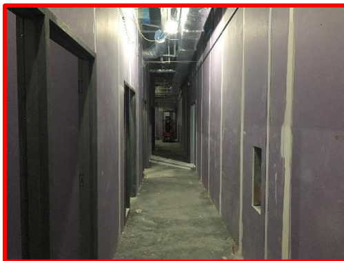
Picture 6: Drywall in the East Admin Area Corridor
