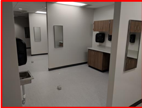
Picture 1: Dental Assisting Lab Ready for Installation of Dental Equipment
