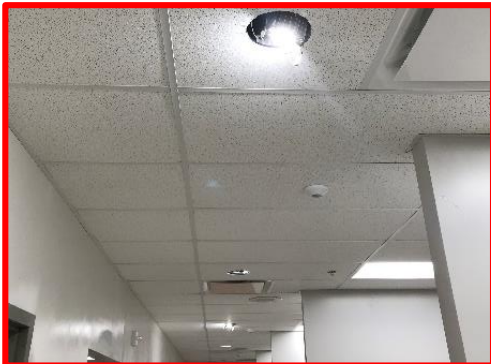
Picture 2: Ceiling Tile in the Dental Assisting Lab
