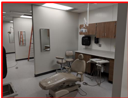
Picture 2: Equipment Installation in the Dental Exam Area
