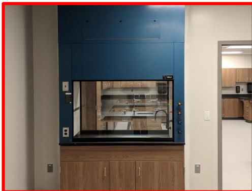
Picture 2: Fume Hood in the Chemistry Lab/Science Prep Area
