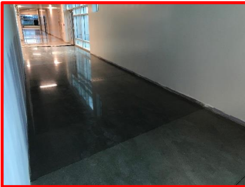
Picture 4: Stained Concrete in Corridor 1003
