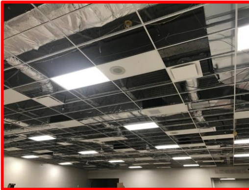
Picture 1: Overhead Devices in the LGIA
