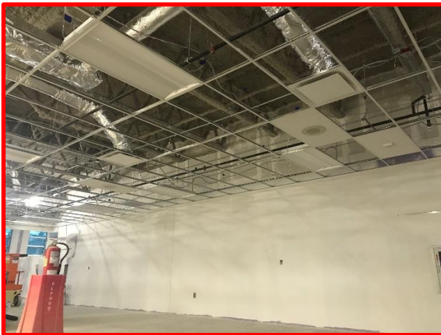
Picture 4: Lights and HVAC Devices in the Learning Commons
