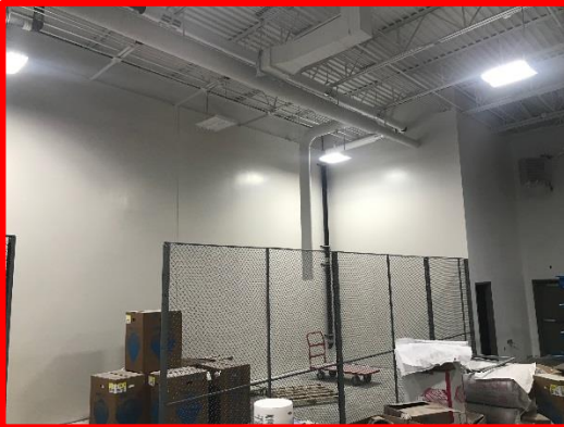
Picture 2: Wire Mesh Partition and Prime/First Coat of Paint in Fire Service Tech
