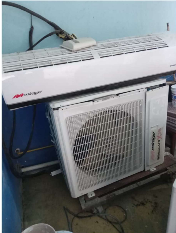
NEW AC UNIT
