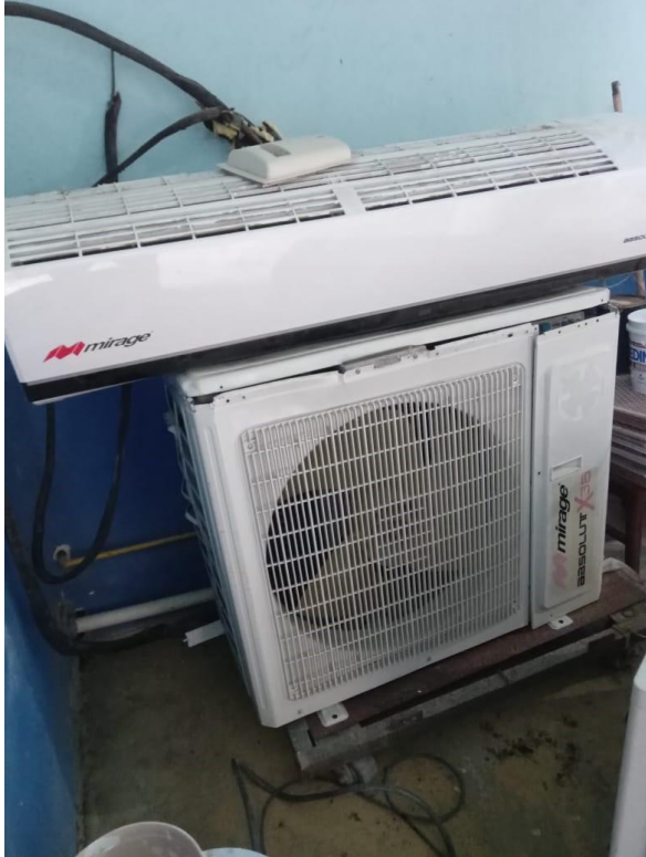
NEW AC UNIT
