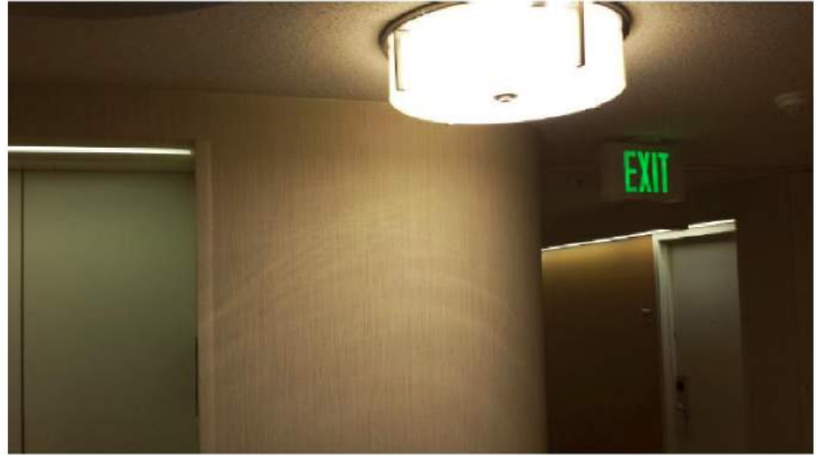
Final look of the fixture mounted in the corridor with new LEDs installed
