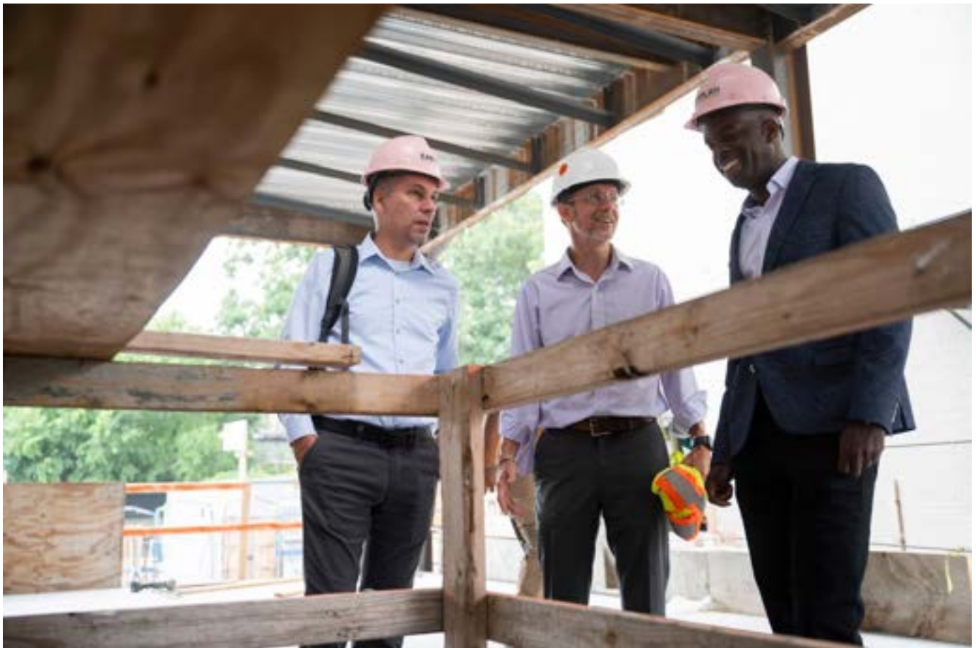
From left, Bill Madsen Hardy, Brian Goldson, both of New Atlantic Development, and Gregory Minott (right) of DREAM Development, talked while on the construction site of a building by the New Atlantic/DREAM Collaborative Development Team in Nubian Square. VINCENT ALBAN FOR THE BOSTON GLOBE
