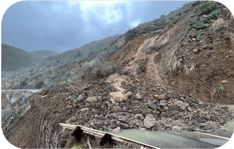
Landslides and Debris Flows
