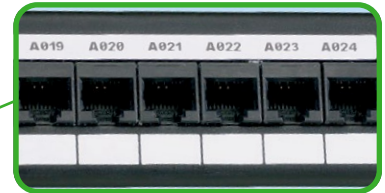
Patch Panel / Face Plate Labels
