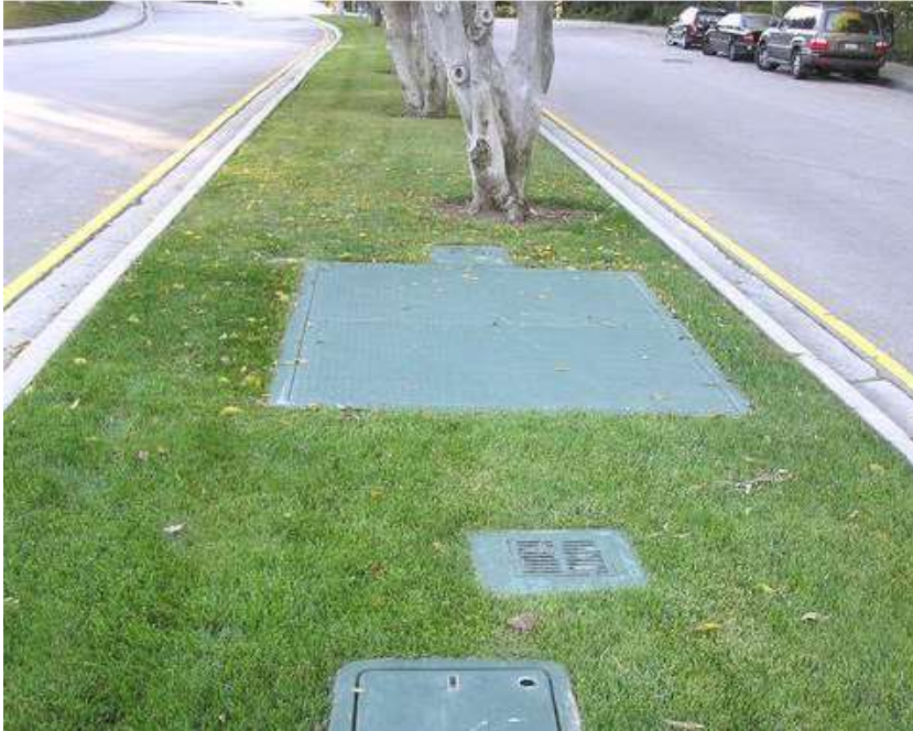
Underground Communication Vault
