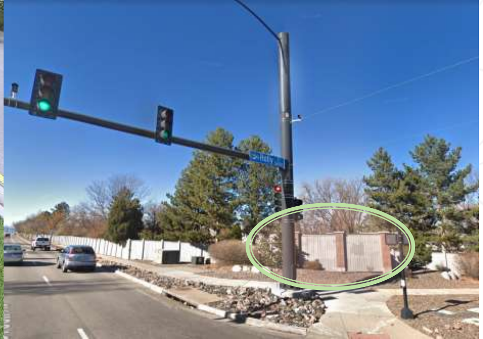
Concealed Equipment Enclosure
