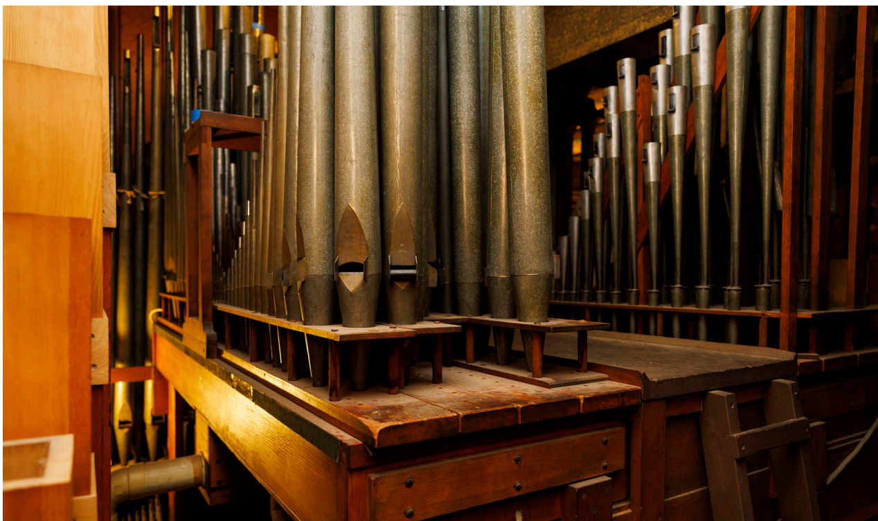
Metal and wooden pipes sit in the organ chamber several stories above the chancel at the Chicago Temple Building. The organ was installed the same year the Temple opened in 1924 and less than 50% of the instrument is fully functional due to age, deterioration, electrical malfunction and water damage from leaks in the floors above the church.
