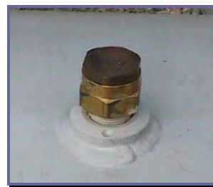
Liquid Withdrawal Valve
