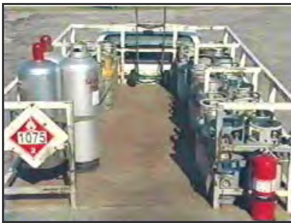
Figure 5.1.6b – Vertically Secured Cylinders
