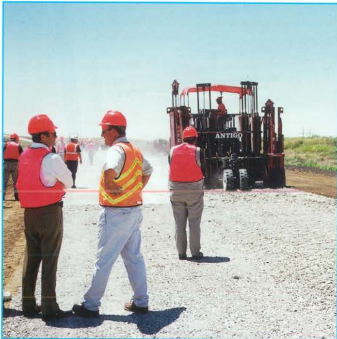
I-76 rubblization project tour, at left, CDOT Deputy Chief Engineer John Unbewust and Project Engineer Jeff Vickers.
