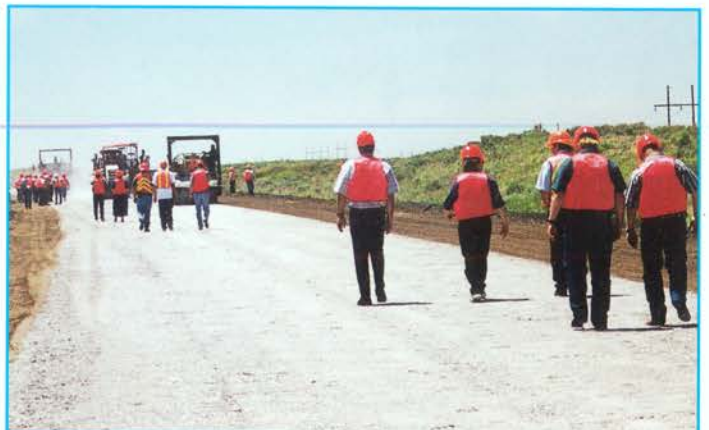
I-76 Project Tour, Phase I - westbound construction, a rubblized roadway, near Sterling Interchange.
