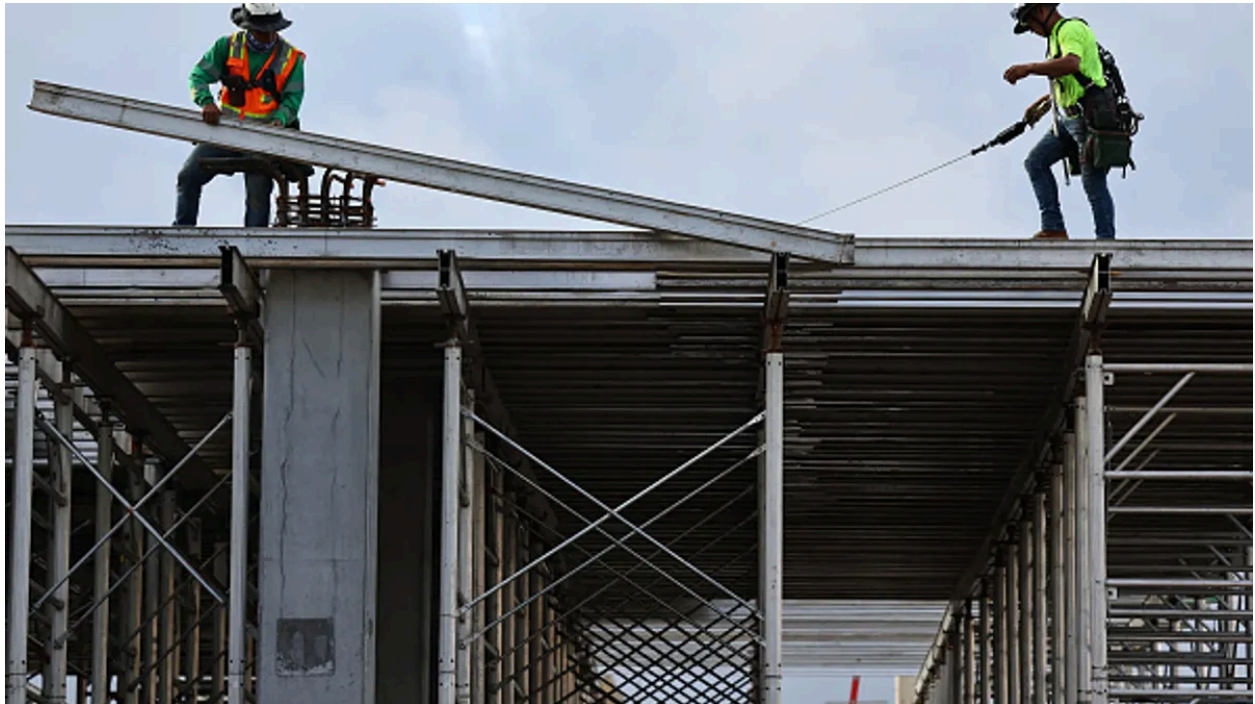
Construction workers help build a mixed-use apartment complex on January 25, 2024 in Los Angeles, Calif. Mario Tama via Getty Images
