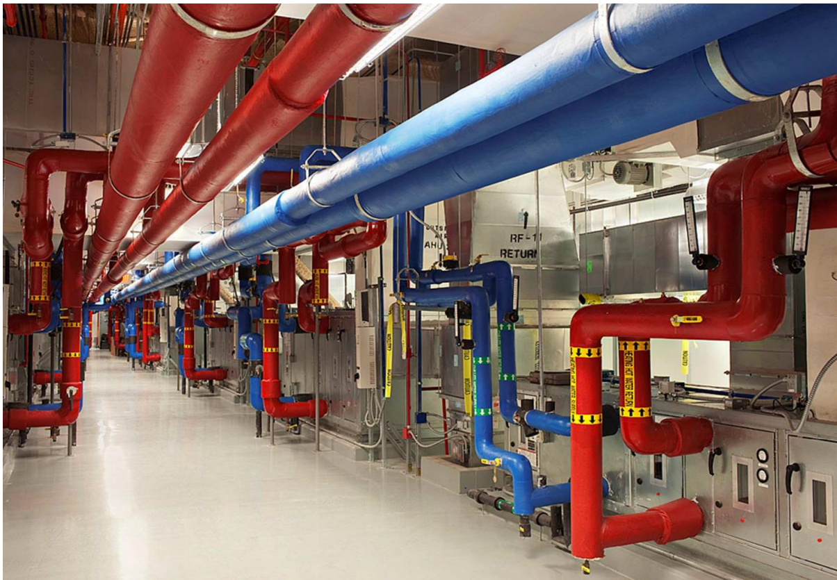
Existing WCDC Phase 2 Mechanical Mezzanine
