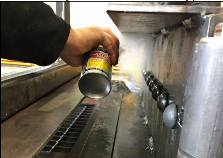
To ready the fixture for re-use, Blaster penetration catalyst is sprayed on both sides of the fixture to loosen rivets without damaging the fixture
