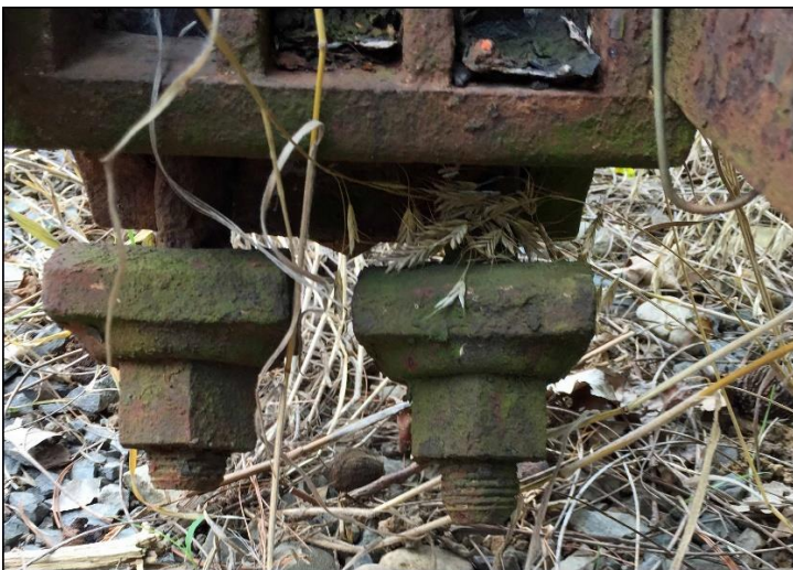
Lower chord cast iron bolted diagonal connection with cast iron washers that have been formed to fit the curve of the cast iron assembly (see photo at right)
