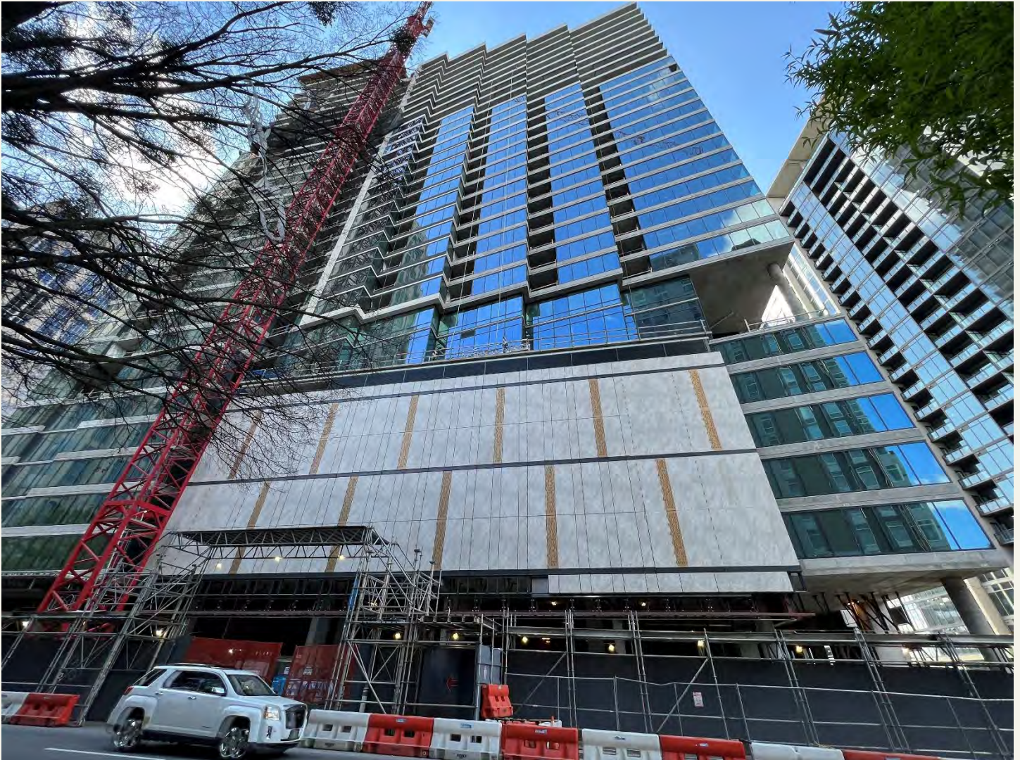
Description: East Elevation of the Site– Exterior Glazing and Elastomeric Coating in Progress.
