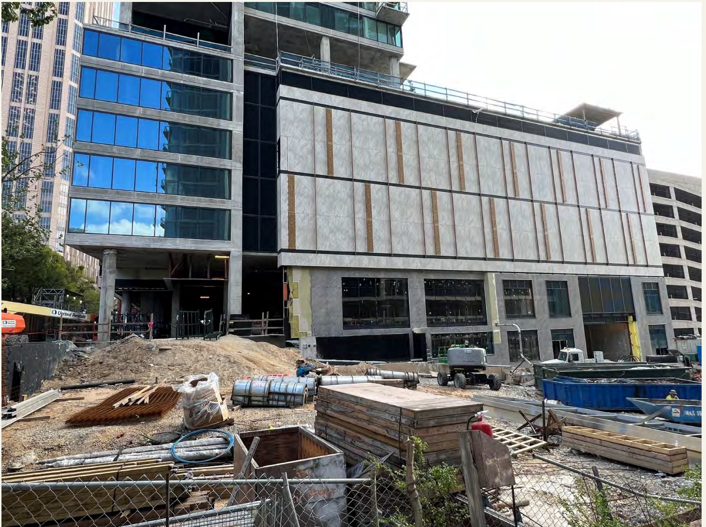
Description: North Elevation of the Site – Exterior Tile/ Facade work in Progress.
