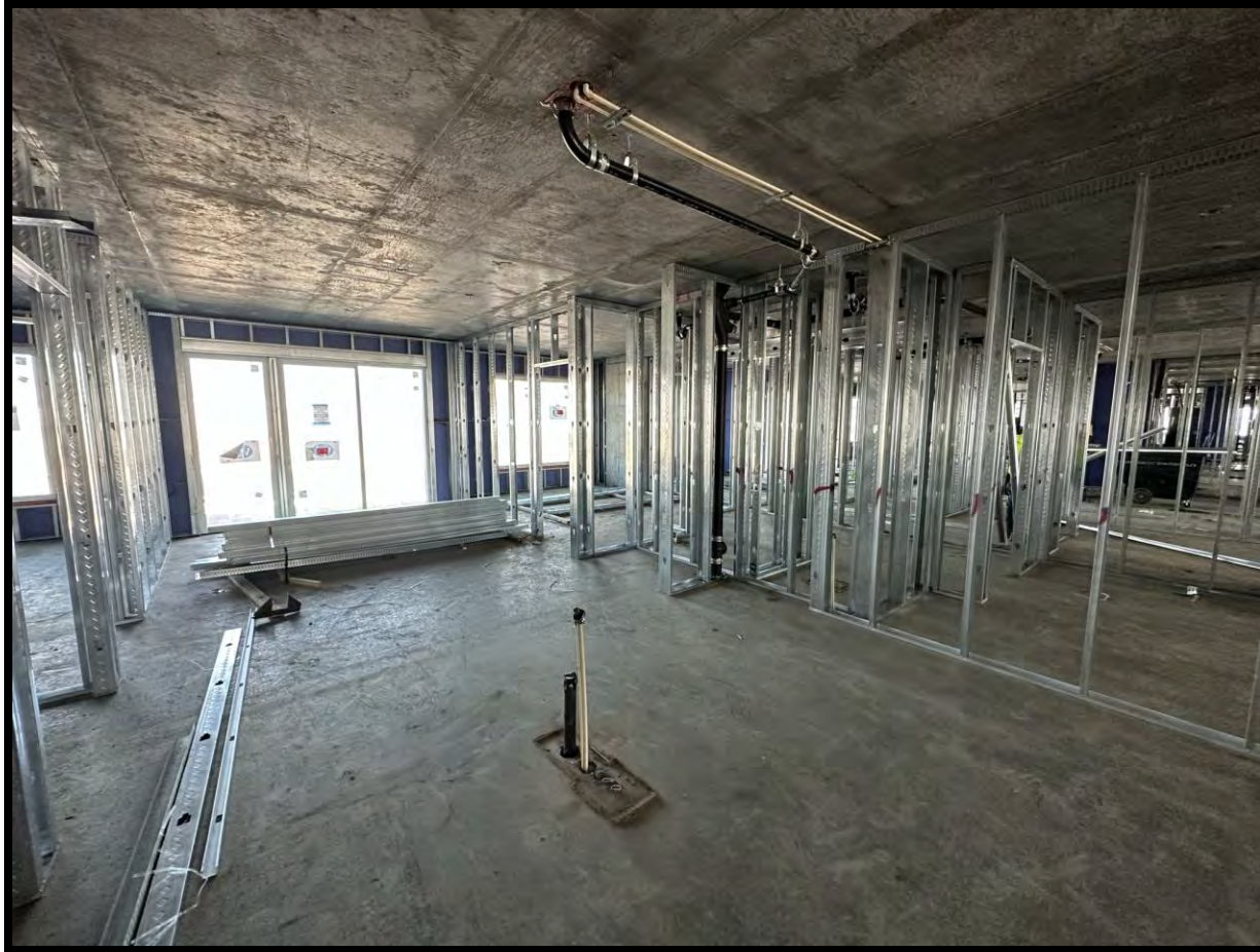
Photo Date: 03/24/2023 Location: Level 10 Units Description: Unit Interior framing is ongoing. (Levels 10)
