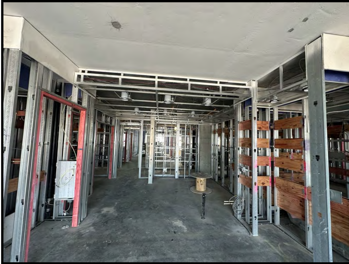
Photo Date: 03/24/2023 Location: Level 12 Units Description: MEP Rough in is ongoing. (Levels 11-14)
