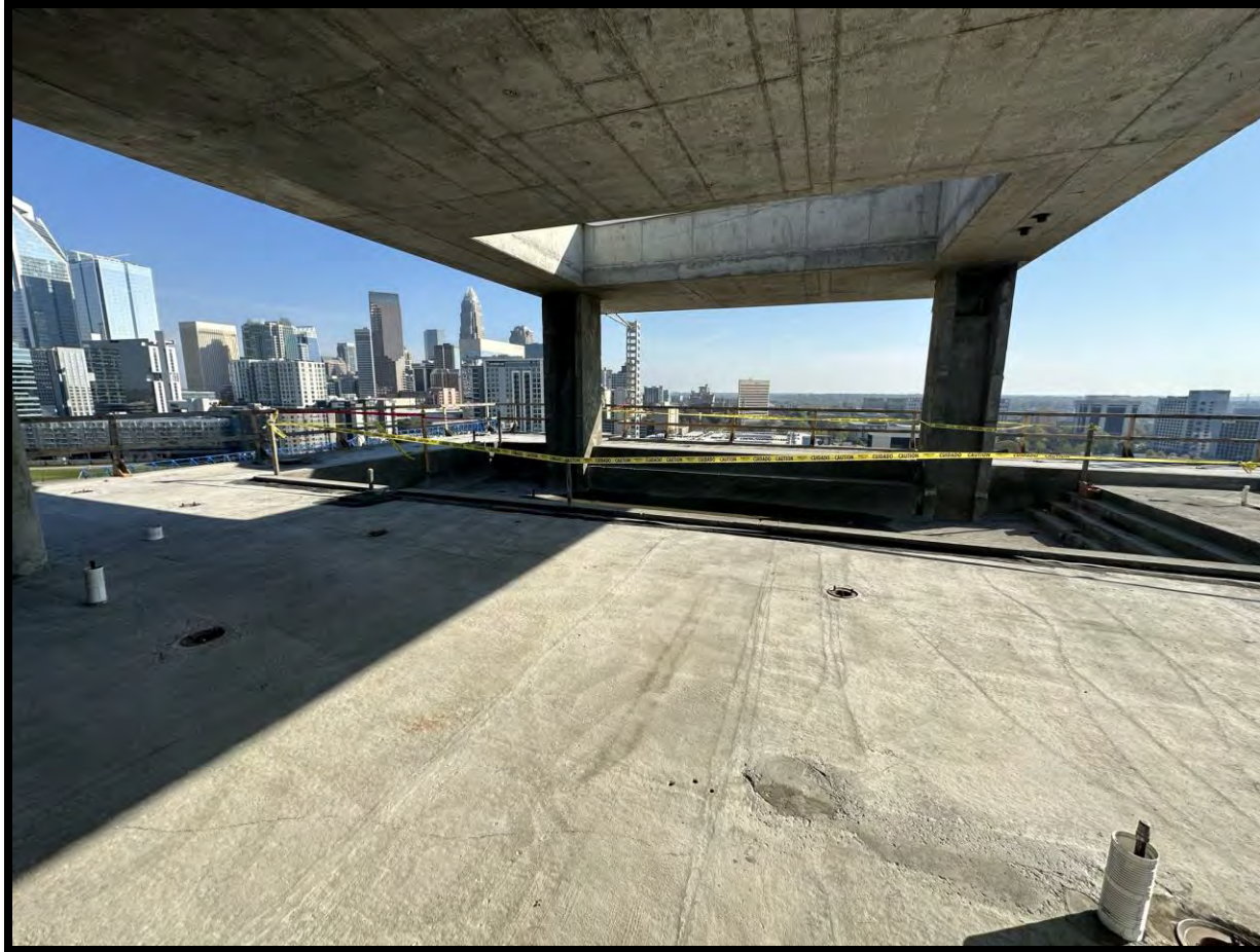
Photo Date: 03/24/2023 Location: Level 16 Pool Deck Description: Pool Deck Prep is ongoing.
