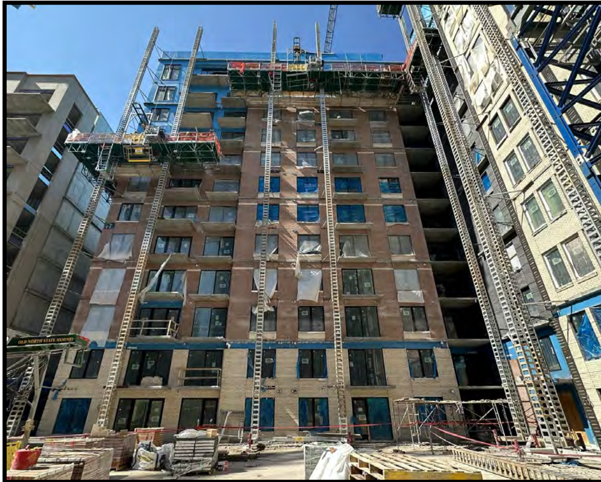
Photo Date: 03/24/2023 Location: Level 4 Courtyard (West) Description: Brick installation is ongoing. (Level 11-15)
