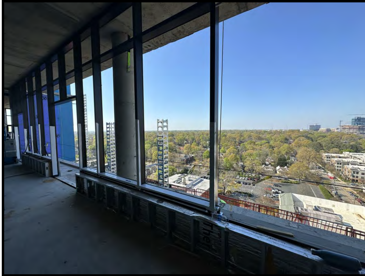
Photo Date: 03/24/2023 Location: Penthouses West Side Description: Window Wall installation is ongoing.
