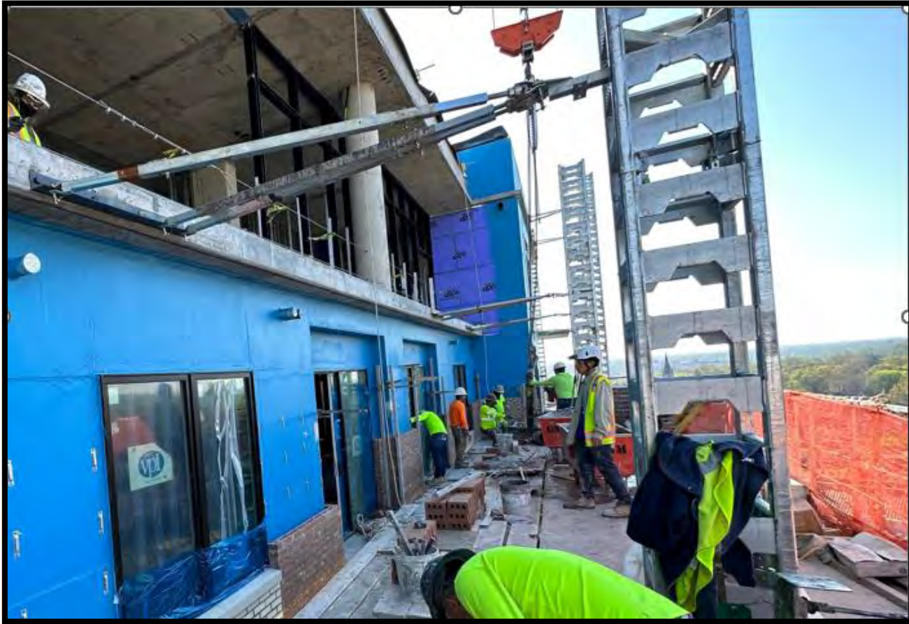
Photo Date: 03/24/2023 Location: West Elevation From HydroMobile (Level 15) Description: Brick installation is ongoing. (Level 15-16)
