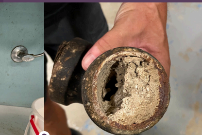
HS plumbing is original and beyond repair. Pipes are clogged and urinals overflow often.
