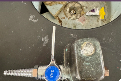
HS science classrooms are cramped, labs are outdated, and gas lines are inoperable for experiments.
