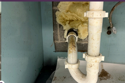
Plumbing under the FACS room sink (pictured) is beyond repair. Six plus years ago, a company cut through the wall to access and clean the pipes during a 2-3 month process to make repairs at each station.
