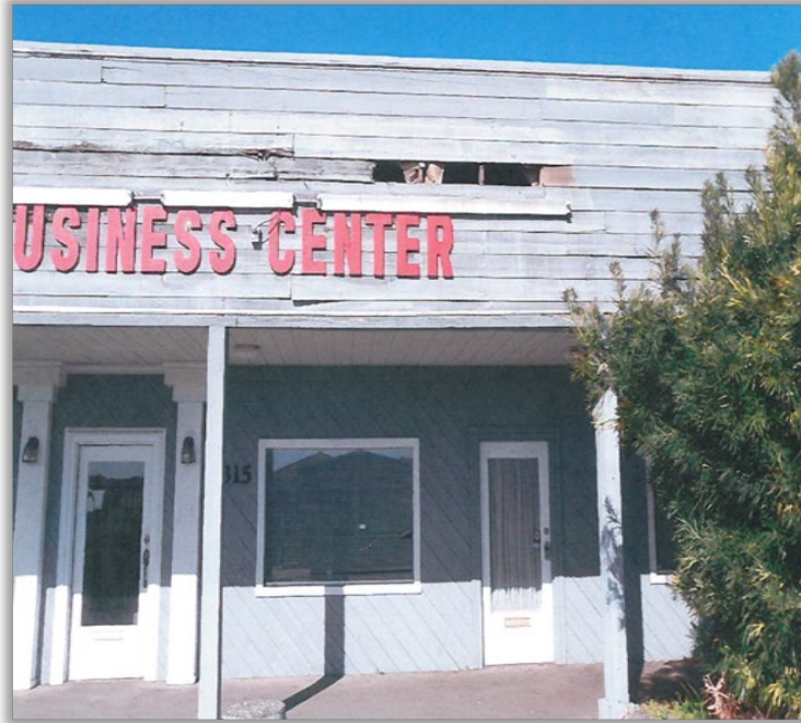
Store Front deteriorating
