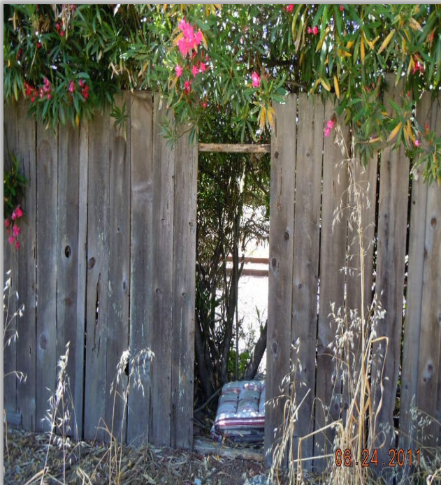
Damaged Wooden Fence
