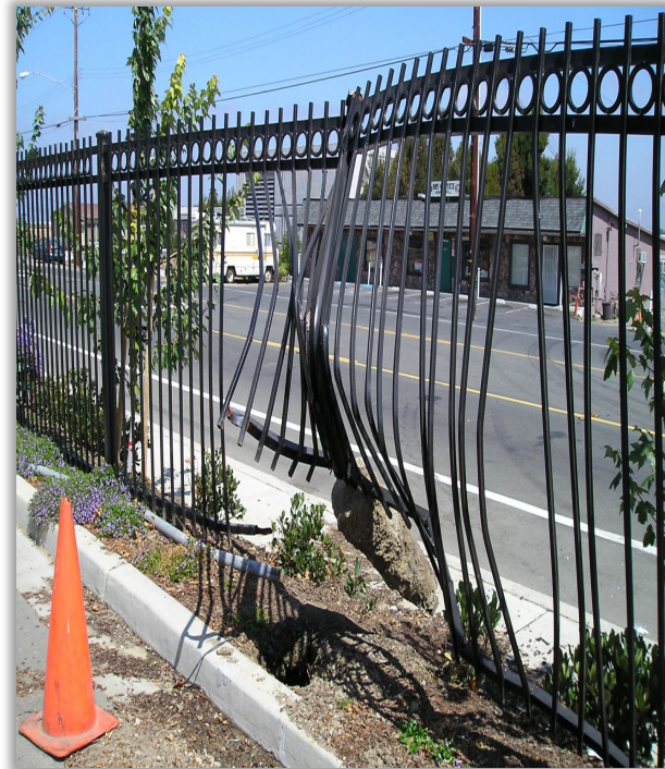
Damaged Metal Fence
