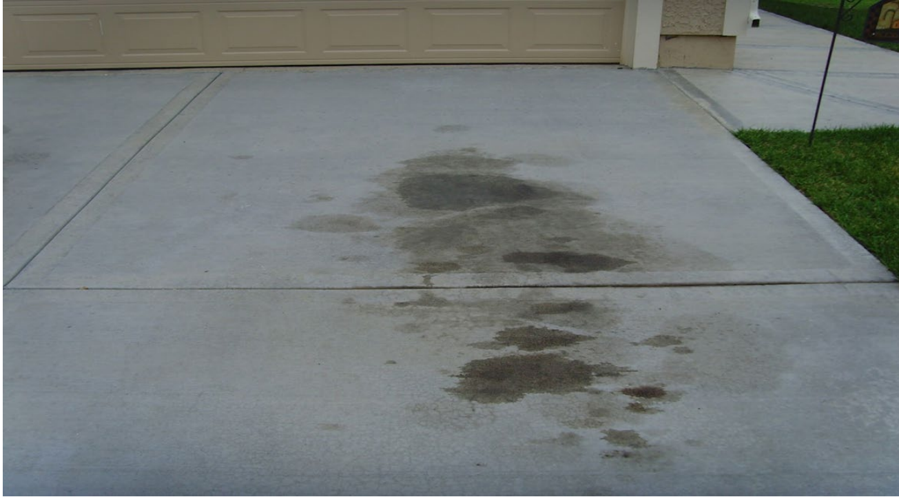
Oil/Grease on the Driveway
