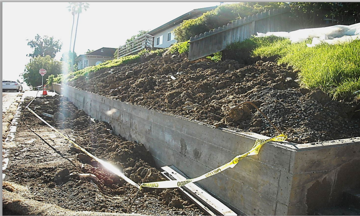
Accumulated dirt in front yard
