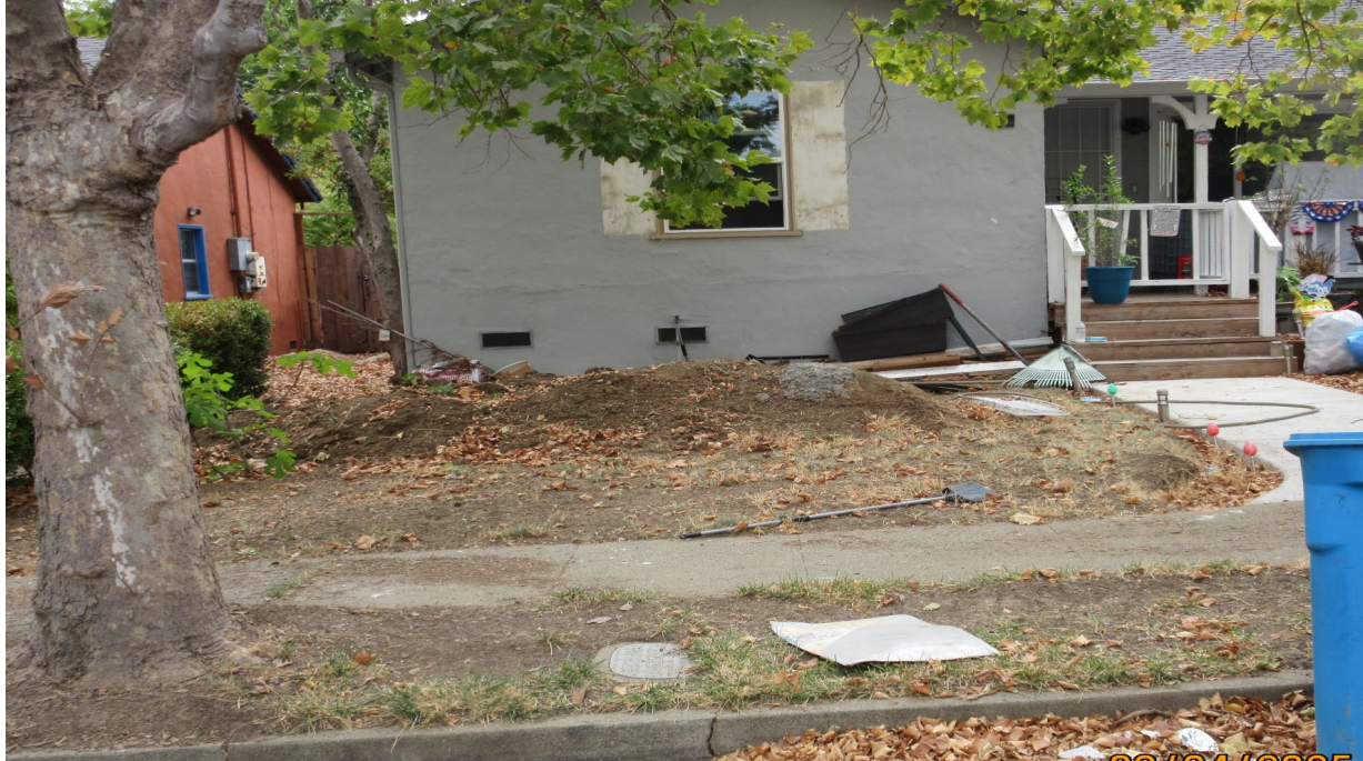
Concrete/Gravel in Yard
