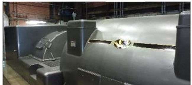
Figure 3: CHP Unit 8 (Source: University of Missouri)
