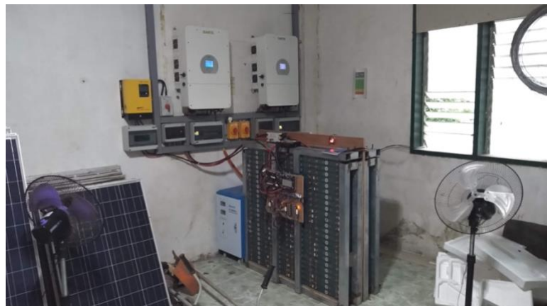
Solar electric generating and storage system providing resilient utilities to St. William's, Paracelis
