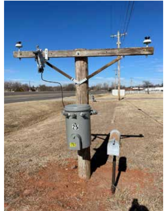
The OMPA Crew at Marlow built this unique mailbox. It is similar the mailbox at OMPA's Fairview office.
