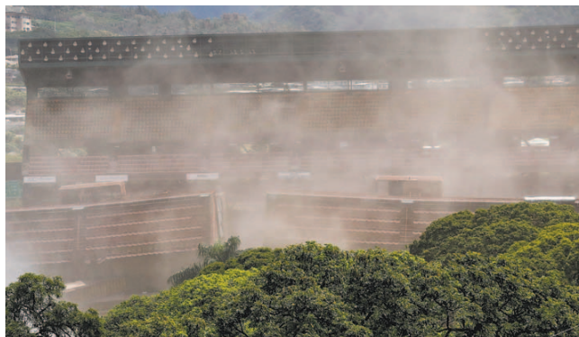
The entire makai section of Aloha Stadium, including the press box, was demolished during this phase using a “rollover” maneuver executed by Hawaiian Dredging Construction Co. and Aloha Halawa District Partners.
