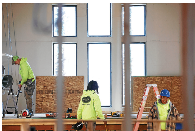
Dallas Rucker, 18, center, and Myia Rex-Dean, 24, gather their toolbelts for more renovations.
